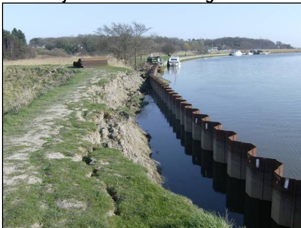
Eroded road with new piling
