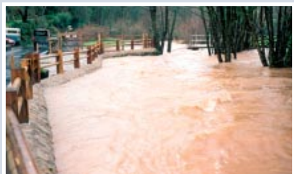
▲ High flows in the River Harbourn contained by the new wall alongside Bow Road
